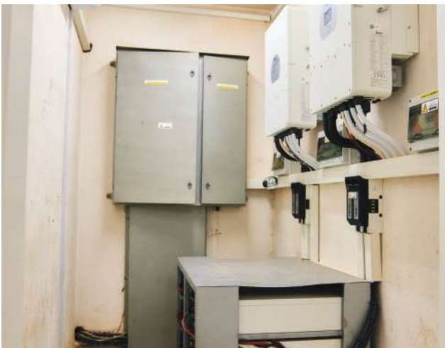
Solar Batteries and Inverters at New Head Office Building
